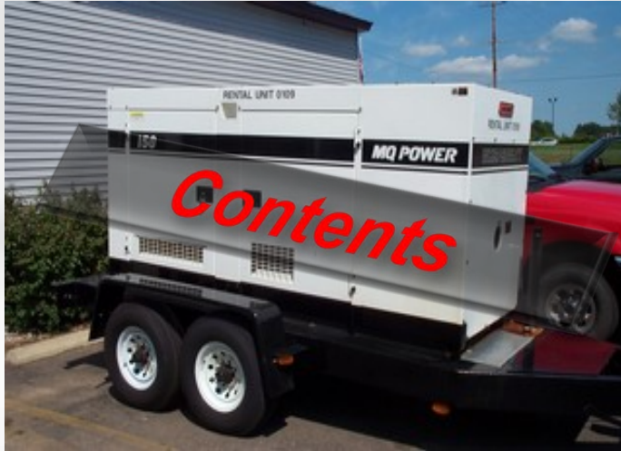
Generator: sitting on a portable flatbed trailer
