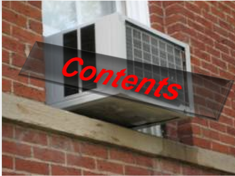
Window HVAC Unit
