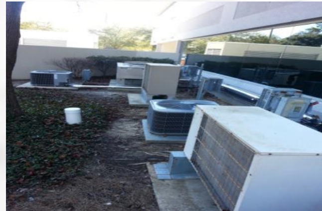
These small condensing units are all within 20 feet of scheduled building and has an ACV < $50K.
