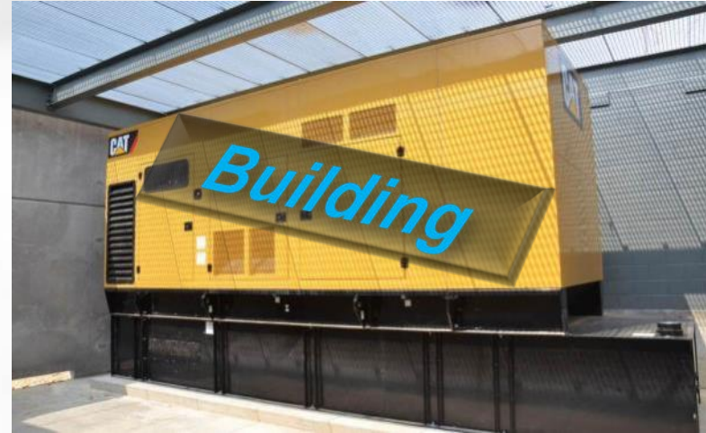
Generator: mounted inside a Permanent Building
