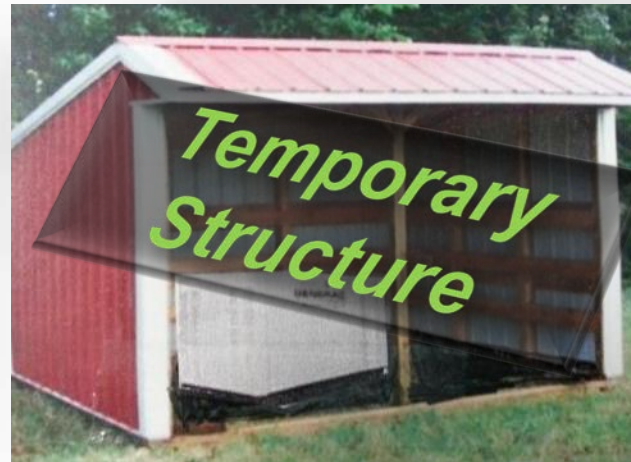
Generator: permanently mounted inside a temporary structure (one with slab floor)
