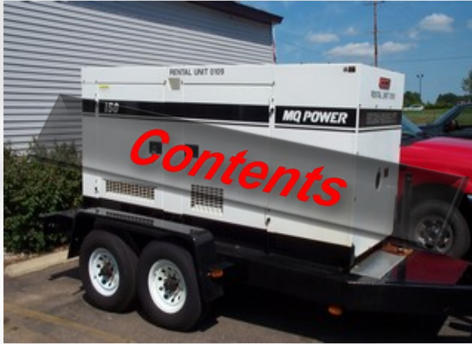
Generator: sitting on a portable flatbed trailer
