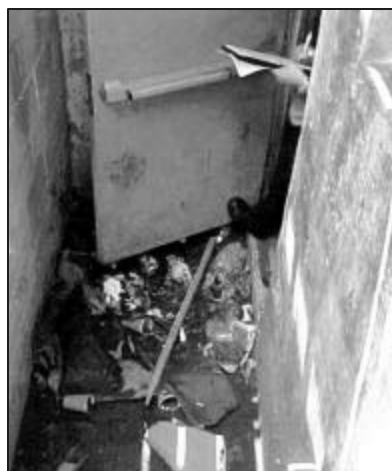
Keep clutter out of exit door pathway
